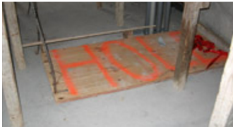
Floor hole cover- Marked hole
